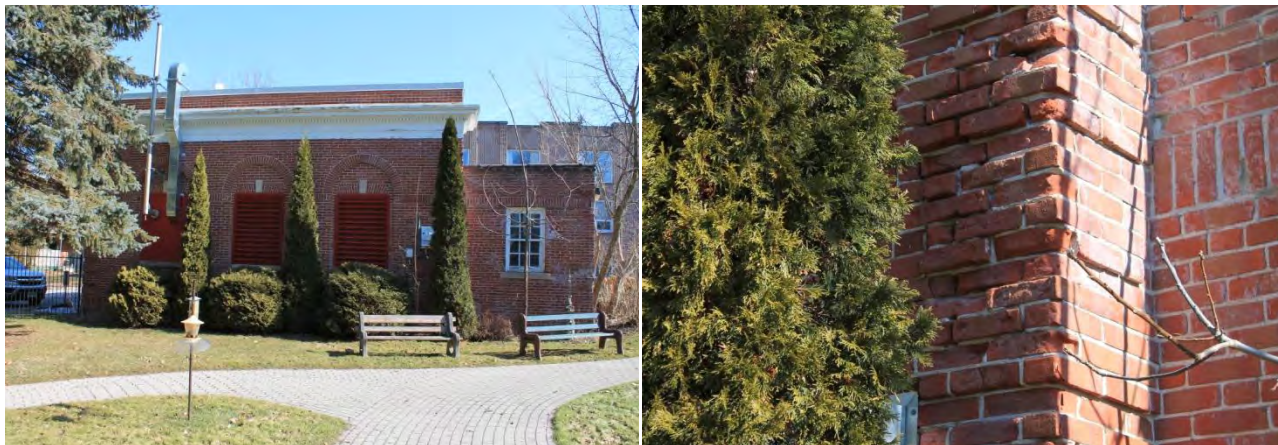
Figures 58 & 59: (left) View of west elevation, looking east (right) Detail view of south corner of west elevation noting damages to masonry (Source: MHBC, 2018)
