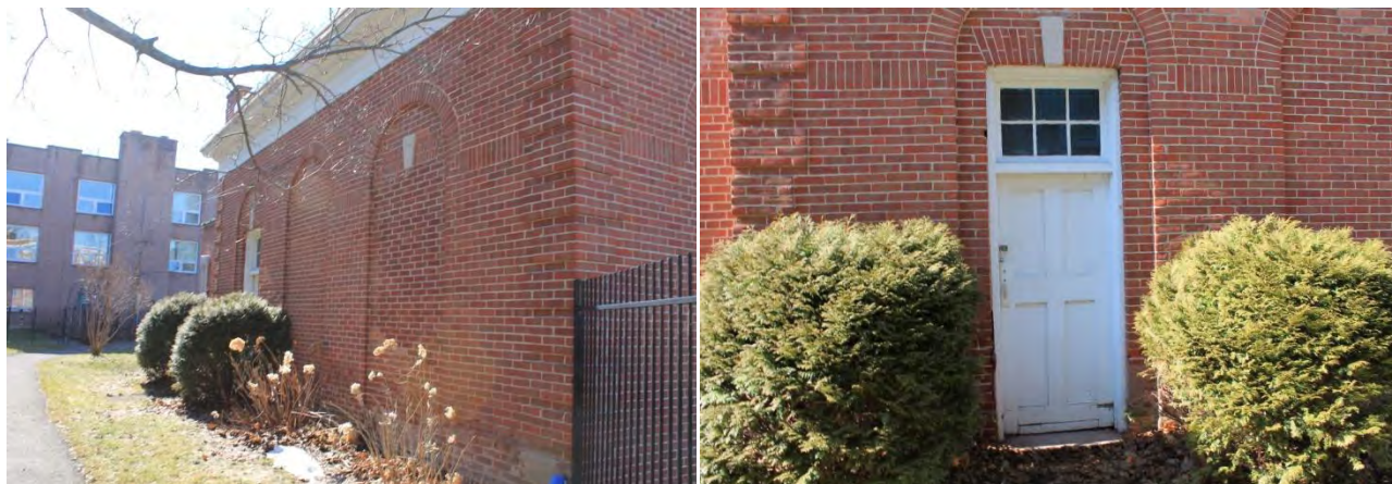
Figures 54 & 55: (left) View of east elevation, looking south (right) Detail view of door at south end of east elevation, (Source: MHBC, 2018)
