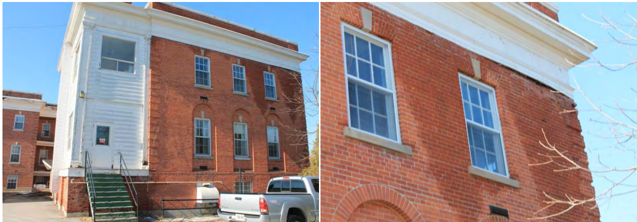
Figures 32 & 33: (left) View of east elevation, looking west (right) Detail view of stringcourse and windows at second storey of east elevation, (Source: MHBC, 2018)
