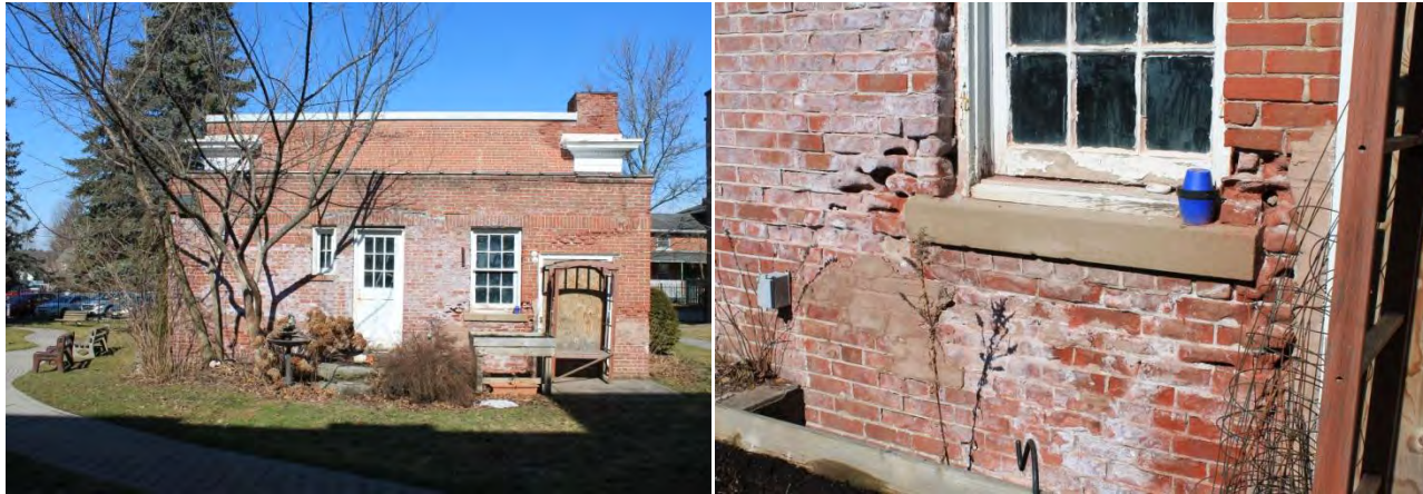
Figures 56 & 57: (left) View of south elevation, looking north (right) Detail view of bricks at south elevation noting damage to masonry (Source: MHBC, 2018)
