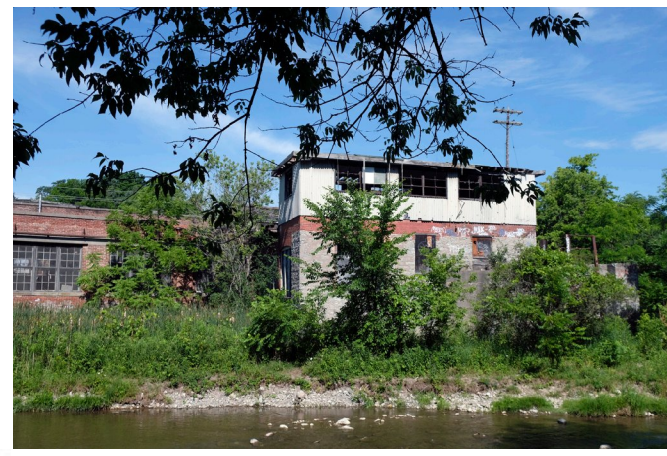
1850-1889, East elevation overlooking river, ground floor stone and brick walls incorporating part walls from original 1850s mill, window openings with multi lite windows, side wall returns to buildings 2 and 4. (encourage preservation of associated mill race and remnant dam structures and interior wood heavy timber structure, remand of 1850s mill)
