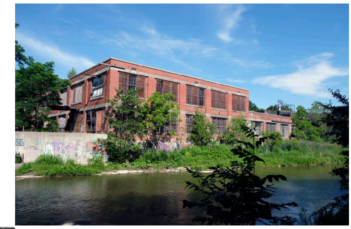
1902, East elevation overlooking river, 2 storey brick walls with concrete banding and wall cap, expressed pilasters, 6 part multi lite windows in 5 window bays with concrete lintels and sills
