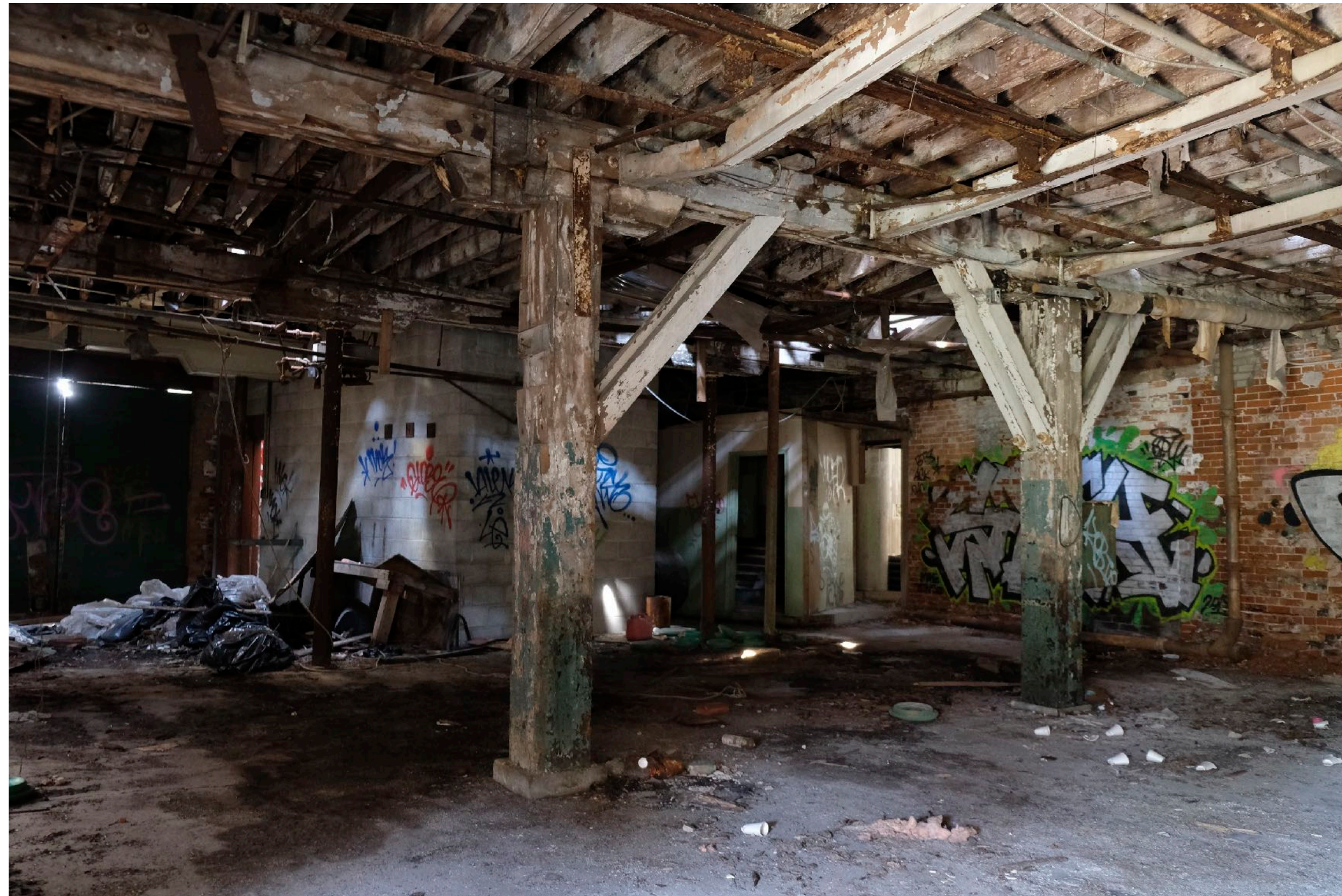
The interior of building 3, the Beamish mill area. The structure is mass stone masonry exterior walls with a heavy timber frame and wood second floor. Rotted wood needs to be removed while the primary frame could be retained, reinforced and jacks added and braced as part of a retention strategy.
