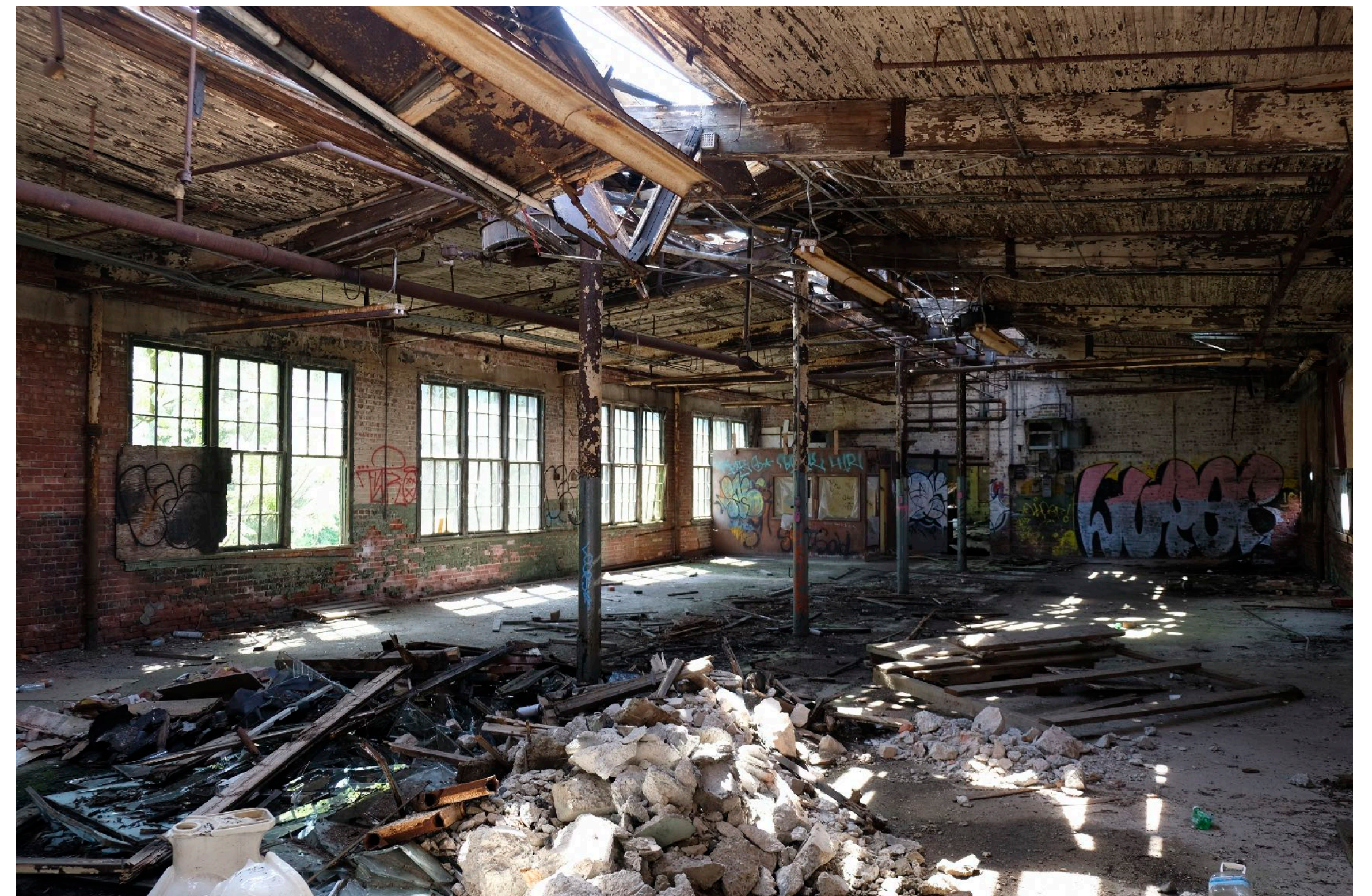
The interior of building 4. The structure is mass masonry exterior walls with a primary steel frame and wood second floor. The wood needs to be removed while the steel could be retained and braced as part of a retention strategy.
