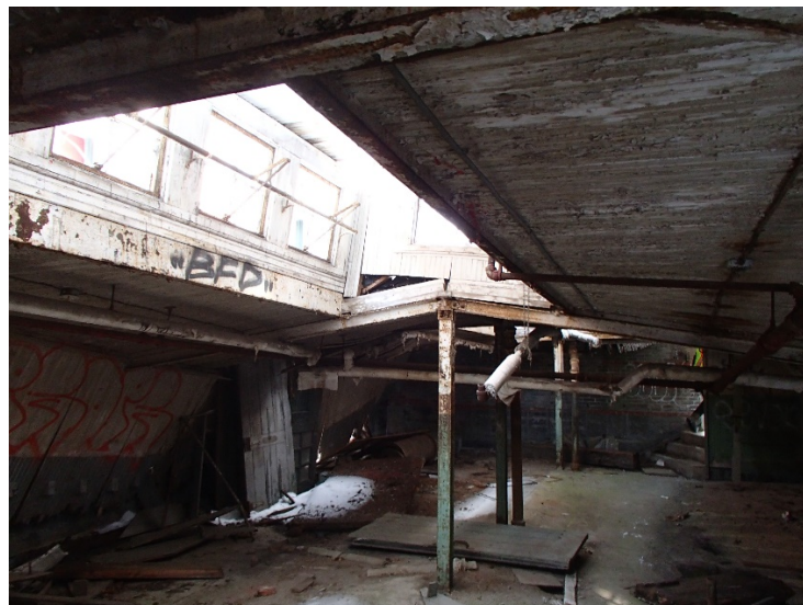
Photo 6: Collapse in Courtyard Area Building, Block #3
