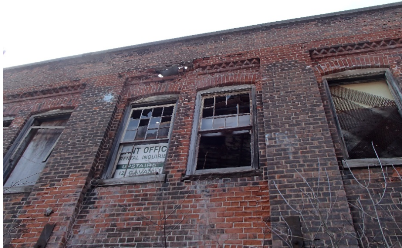
Photo 5: Parapet Deterioration East Wall, Block #2
