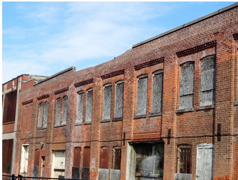
Photo 4: Parapet Deterioration and Wall Bowing, West Wall, Block #2
