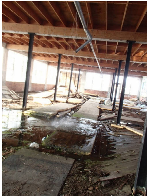
Photo 8: 2 nd Floor Level Looking up at Underside of Roof, Roof Drain Pouring into Building – Block #5
