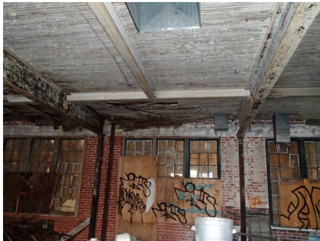
Photo 2a: 2 nd Floor Deck Collapse in Block #1
