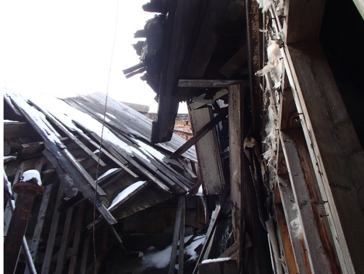
Photo 3: 2 nd Floor and Roof Collapse, Block #2, Area behind West Exterior Wall
