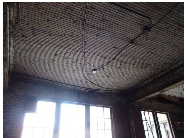
Photo 2b: 2 nd Floor Deck Collapse in Block #1
